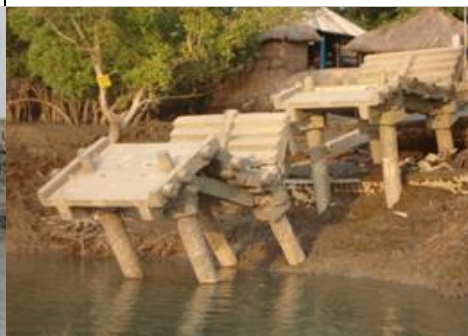
Collapse of concrete jetty due to bank failure in Vidya river
