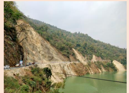
Landslides affecting the alignment of NH-31
