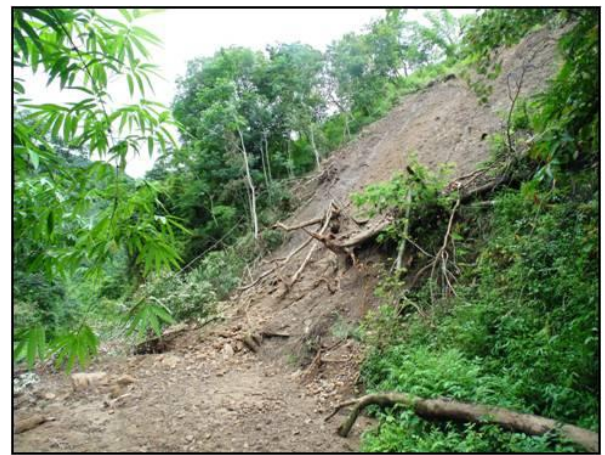
Fig. 5: Photograph showing sectional view of the landslide.
