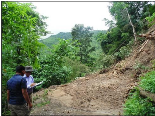
Fig. 6: Photograph showing total road blockage of New Heaven - Lamlang Gate section of Old Imphal - Ukhrul road.
