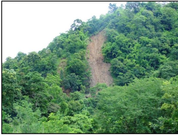
Fig. 4: A view of the landslide along New Heaven - Lamlang Gate section of Old Imphal - Ukhrul road.
