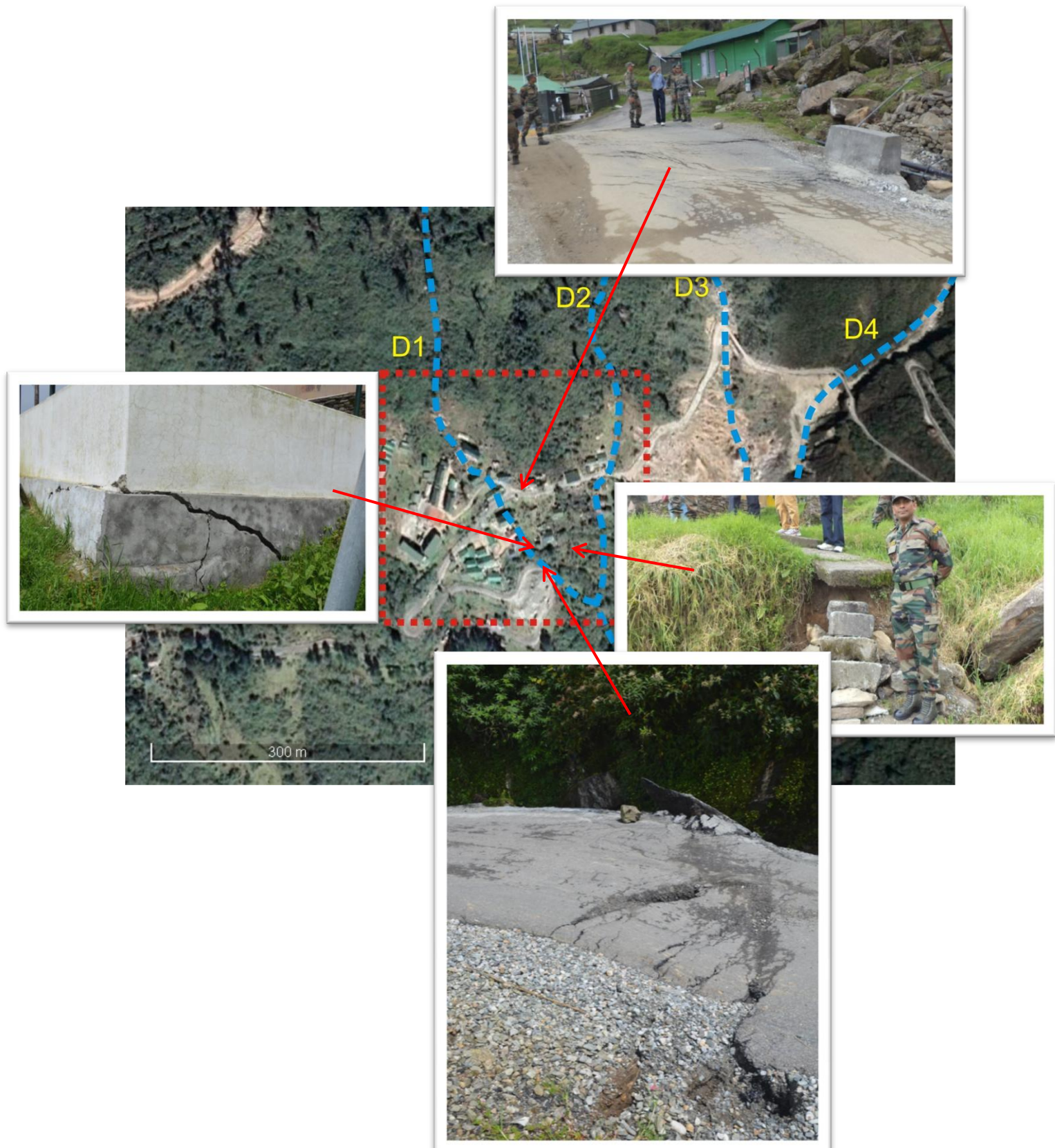
Fig. 5: Photographs showing disposition of surface evidences of active subsidence in the form of cracks developed in the culvert, floor and roads.
