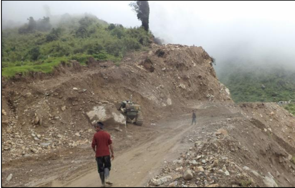
Fig. 3: Unsorted and unconsolidated debris material exposed along the road cutting (JNM axis) ahead of MS-8.
