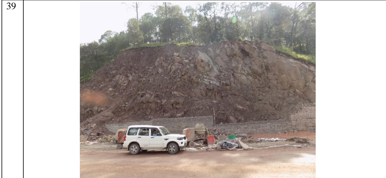
Field Photograph of Slide along NH-22, Chandigarh, Shimla, Road, at RD: 87+480
