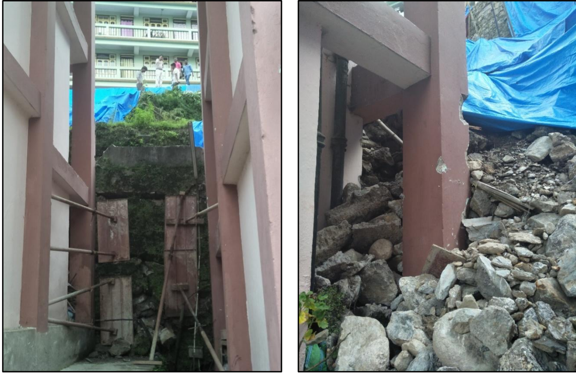
Fig. 3 & 4: The failure affecting the slope and the buildings in Upper Syari.
