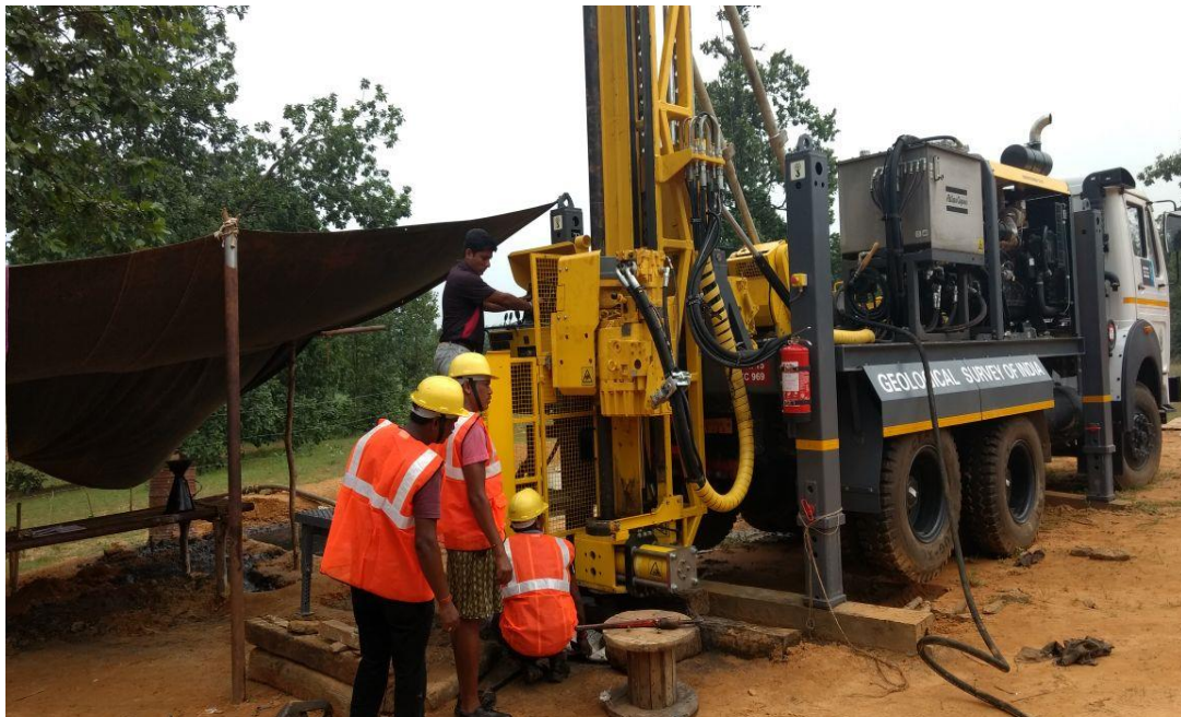
Atlas Copco Product Specialist acquainting the GSI crew with the Drilling M/c at drill site.
