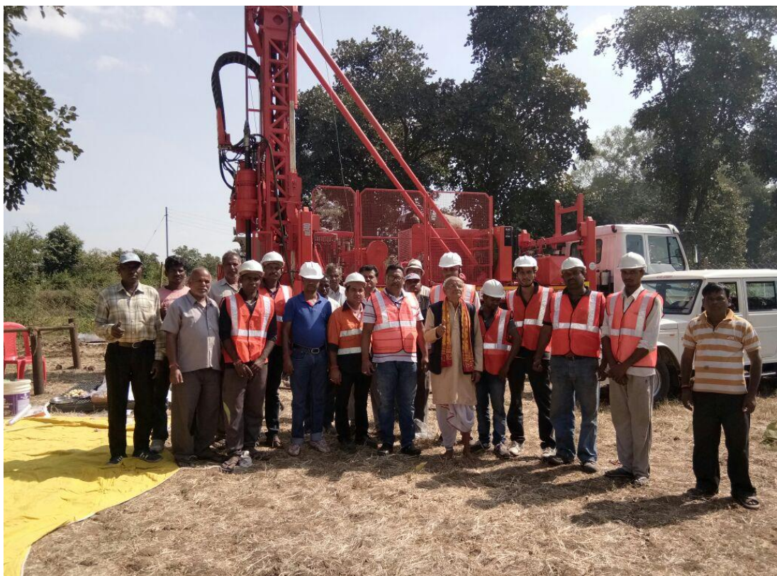
SANDVIK Service Engineer along with the GSI team with the Drilling M/c at drill site.
